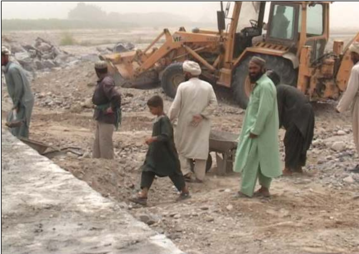
CIDA-funded bridge in Arghandab, Kandahar, Aug 22, 2007 (Child in foreground is filmed lifting heavy loads)
