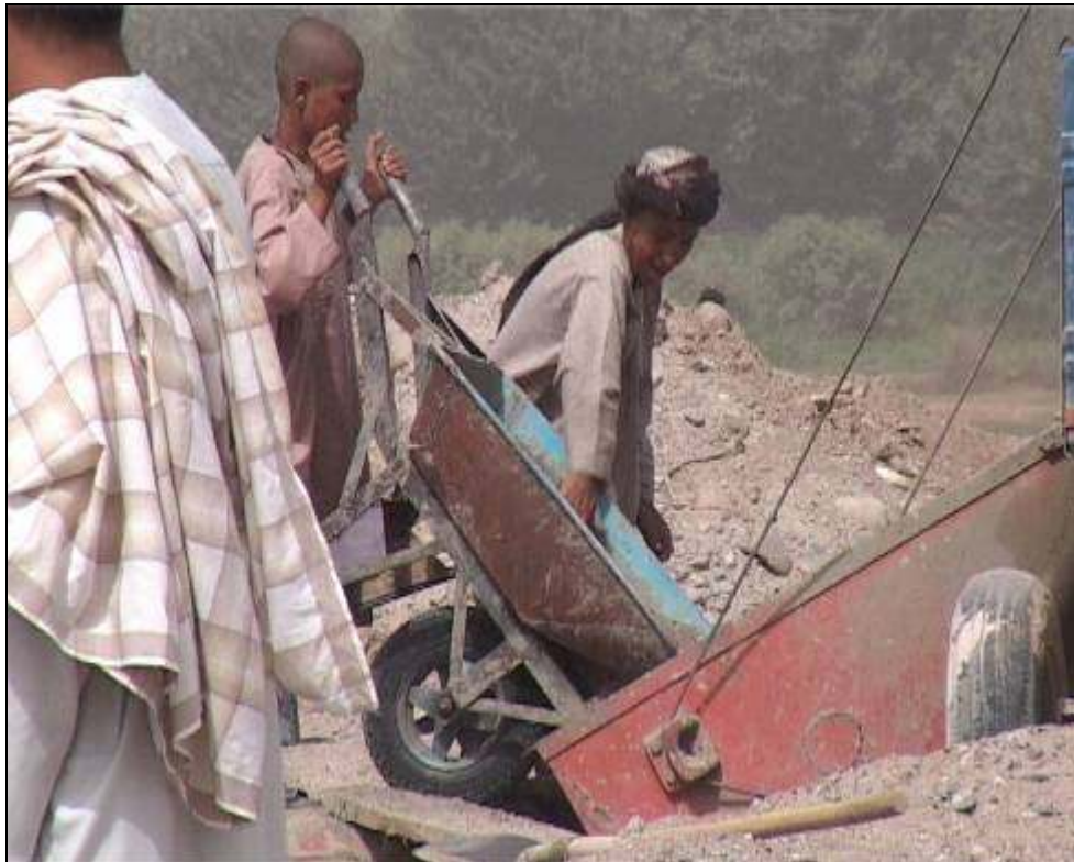
In August 2007 Child labour was seen being used on this CIDA-funded project to build a new bridge in Kandahar.
